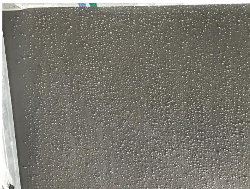
Figure 47: Droplets inside ceiling
