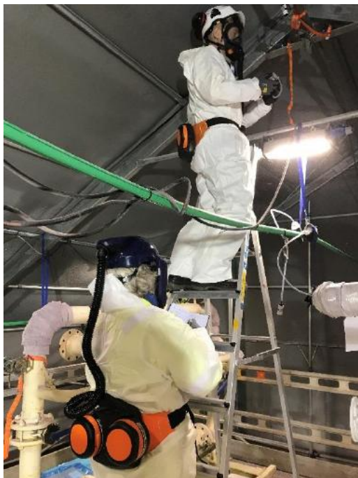
Figure 27: Check of pump flow, ceiling level (C0)
