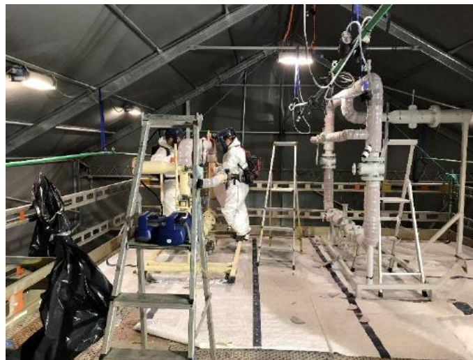
Figure 6: Overview of size of scaffolding work level, including the insulators work area
